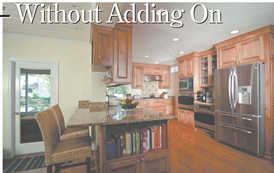
Sun Design Remodeling removed a rear bearing wall in a circa 1955 ranch, co-opting a seldom-used rear porch into an expanded new kitchen. The dining counter is a de facto space divider and a convenient serving station.
