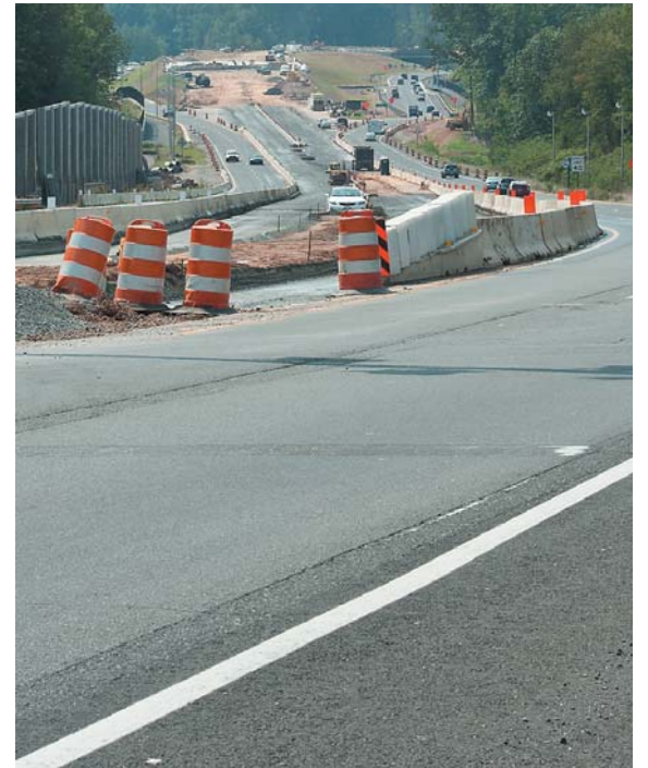
Construction on Fairfax County Parkway in the Fair Lakes area of Fairfax County continues. This image shows the southbound view of Fairfax County parkway from the Route 50 bridge on Aug. 17. The Route 50 bridge is being widened, and two bridges are being built, one over Monument Drive and one over Fair Lakes Parkway.
