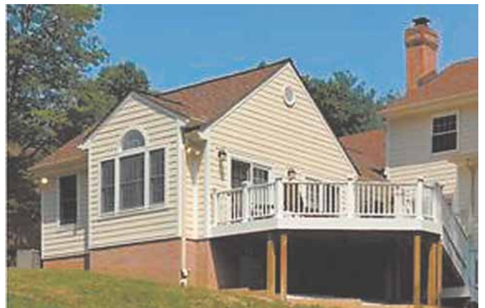
The addition of a main-level master suite with easy access to outdoor living space paves the way for aging in place and family entertaining.
