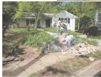
The original front walk — which included stairs in several places — was too steep for Jaime, who now requires crutches to get around the house.
