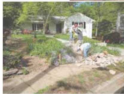
The original front walk — which included stairs in several places — was too steep for Jaime, who now requires crutches to get around the house.
