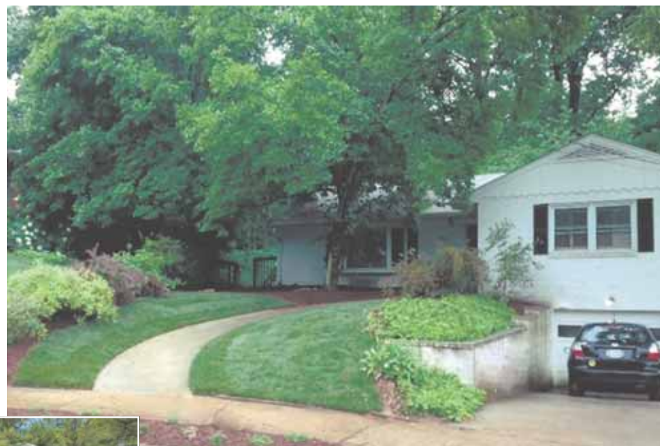
When Jaime Marquez began having difficulties getting from the house to the driveway, Glickman Design Build created a graduated front walk for the Arlington family. The new walk rises one inch per foot. The plan included replacing a front stoop with a "zero step" entry and widening interior doors and halls.
