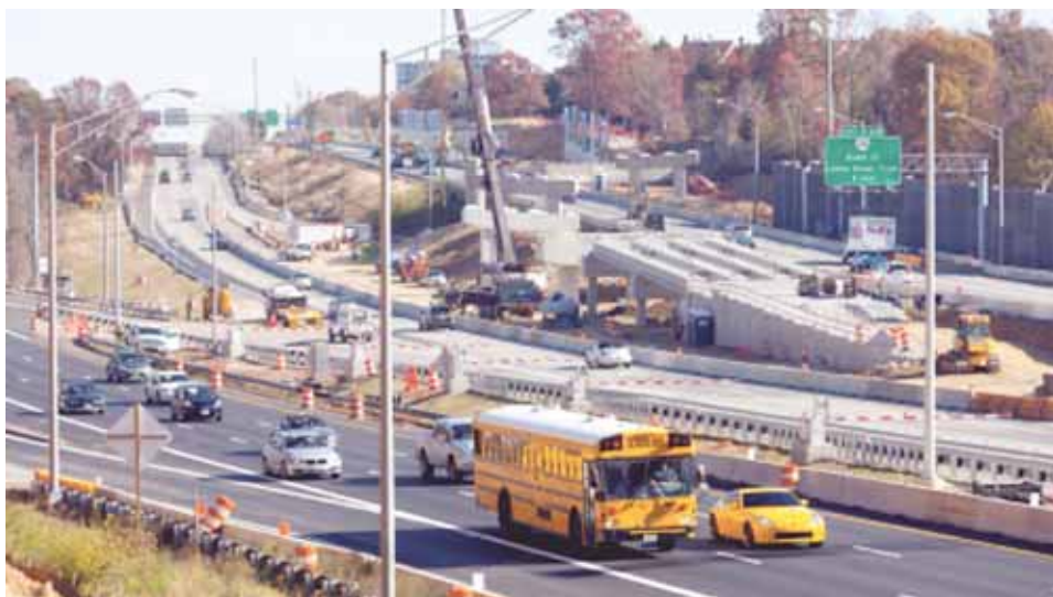
The 95 Express Lanes, scheduled to open in early 2015, will require all users to purchase an E-ZPass. Shown here is construction from fall 2013 at the northern end of the project area.
