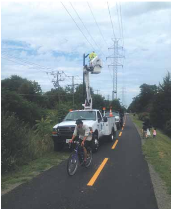
R.E. Lee Electric Co., Inc. was contracted to install lights along the W&OD trail in the Town of Herndon. There are 39 light poles being installed with this phase of the project. A potential future phase of lighting is from Ferndale Avenue to Crestview Drive.
