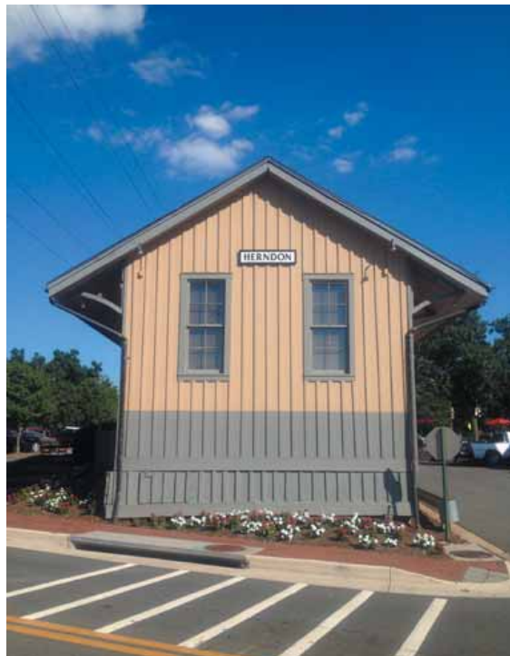
PHOTOS BY RYAN DUNN/ THE CONNECTION In July work was done on the historic Herndon depot building to replace weather damaged board. The depot building was added to the National Register of Historic Places in 1979.
