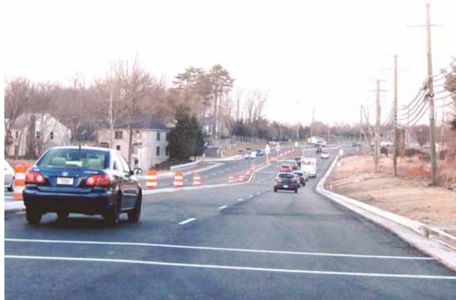
Motorists drive on the two, new northbound lanes of Stringfellow Road, late Monday afternoon, en route to Route 50.
