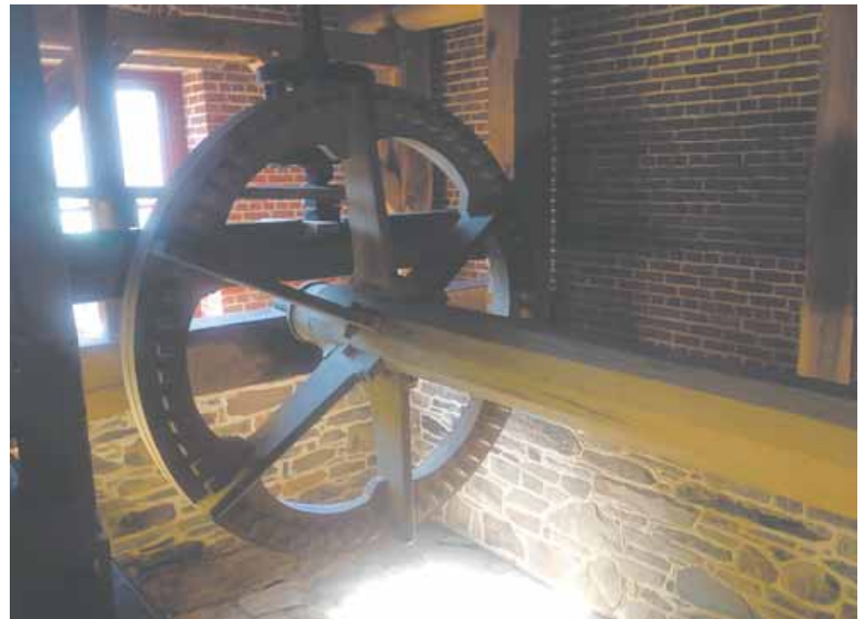
The new shaft which services the Colvin Run Mill water wheel is an oak tree that fell in New York state during Hurricane Sandy in October 2012.
