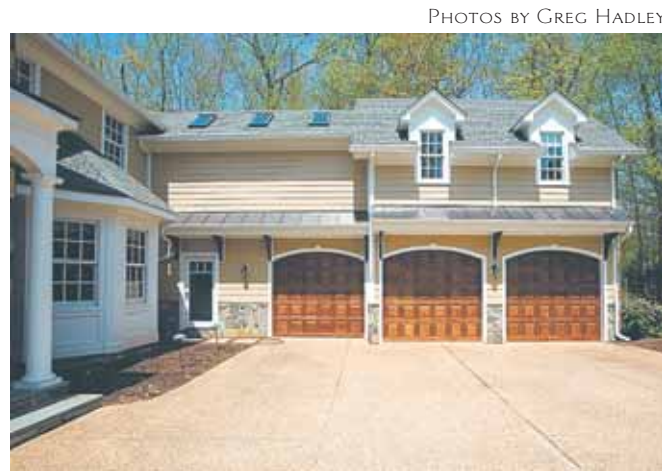
The metal-clad overhang specified by Sun Design provides needed protection from rainfall — which had seriously damaged the previous garage doors.
