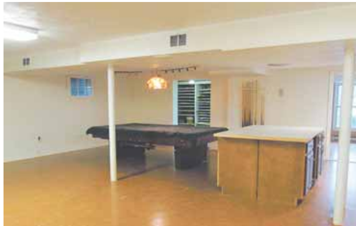
BEFORE: The previous lower level was little more than a partially finished basement that hadn't been used for recreational purposes in years.
