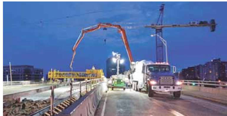
In the over-night hours, crews pour the deck for the Seminary Road bridge over I-395.
