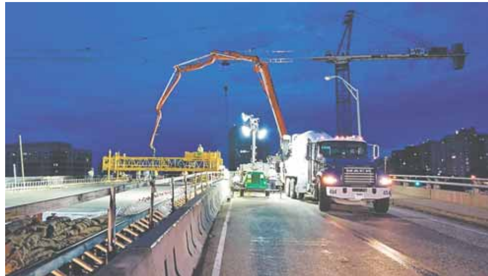
In the overnight hours, crews pour the deck for the Seminary Road bridge over I-395.
