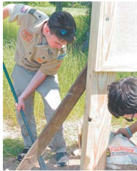
Thomas Pollack says they started on the kiosk at 8 a.m. Saturday morning and spent several hours digging two three-foot holes for the 6 x 6 posts. By 2 p.m. it was 94 degrees and the concrete was being poured. "It won't take long to harden in this heat," Pollack said.
