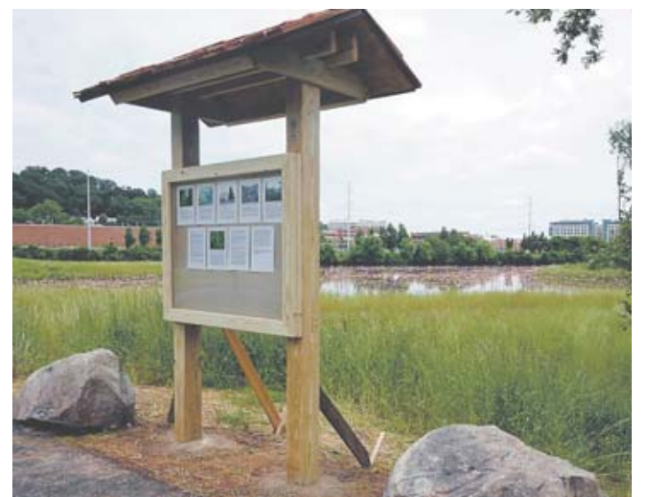
The kiosk designed and built by Troop 135 in Alexandria is finished after a hot day of construction over Memorial Day weekend. It illustrates the Four Mile Run restoration area and will include pictures of birds that frequent the area.
