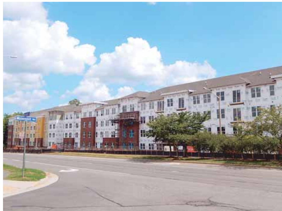
Work is progressing on construction of the Residences at the Government Center, along Monument Drive in Fairfax.
