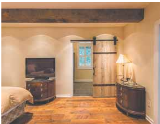
To make room for the larger master suite, Chris Arnold at Foster Remodeling Solutions devised a way to eliminate an obstructive bearing wall by installing an 8” x 17’ steel beam attached to concealed vertical supports. To reinforce the rustic design theme, the exposed beam is wrapped in reclaimed barn board. The floors are also old barn wood milled to specification.
