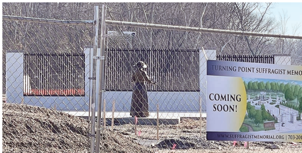
Site of the Turning Point Suffragist Memorial under construction with expected completion in Spring 2021.
