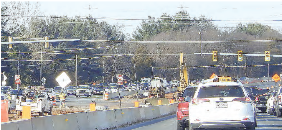
Construction proceeds on Route 28 in Centreville, while traffic packs both sides of the road, during afternoon rush, heading north toward the Old Mill Road intersection.
