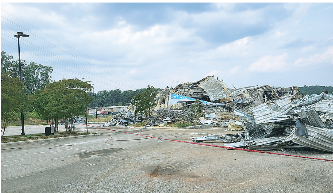
At the site there are piles of debris that were once the office buildings.
