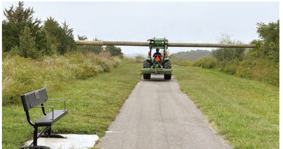
A recycled 50-foot utility pole is moved to the site by maintenance operations employee Alex Guevara-Santos in advance of installation day.
