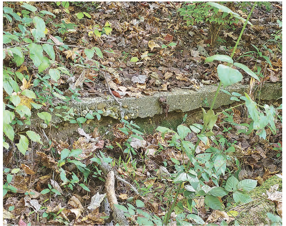
It's not clear what this concrete was. During the 1940s, the Bureau of Public Roads tested asphalt road surfaces at Huntley Meadows
