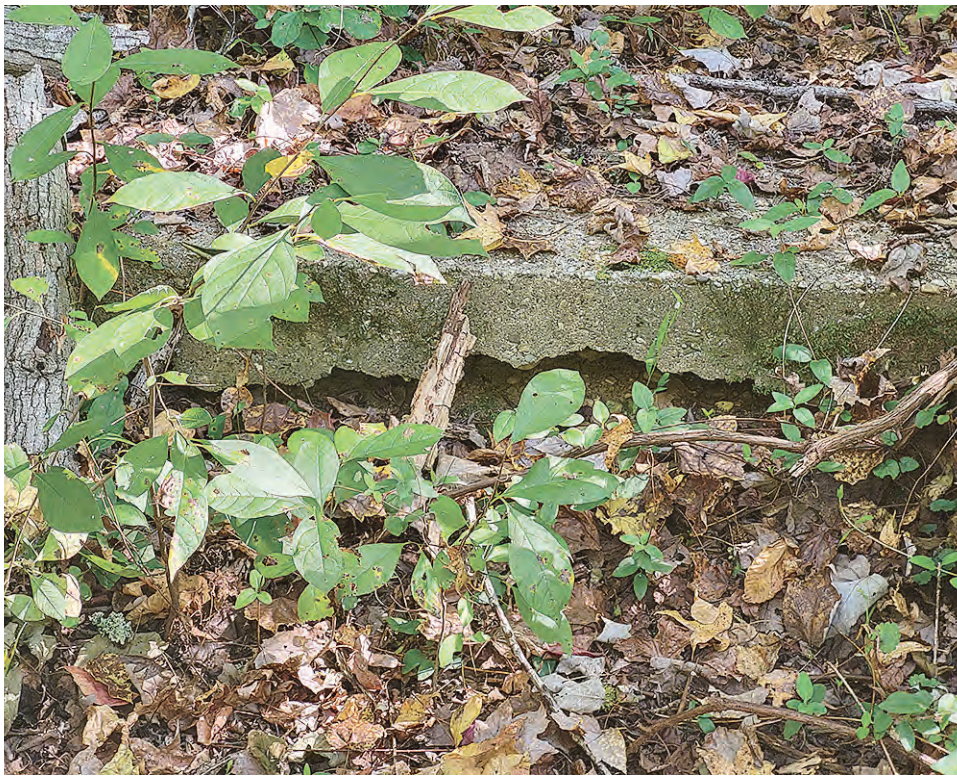
The concrete seems to be under a few inches of soil.
