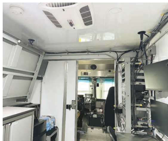
Inside view of a Communication Vehicle (CV), one of 5 deployed as needed to provide longer term connectivity via LTE and/or Wi-Fi, in an air-conditioned command space with overnight accommodation for 2 first responders, with monitors, charging stations, a large exterior screen and speakers for briefings
