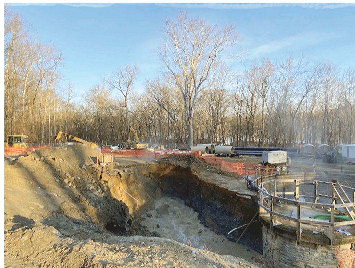
SCREENSHOT VIA LIVE FAIRFAX COUNTY VIDEO, DC WATER.COM Sewage flows in DC Water's Manhole #31 in Great Falls, located approximately a football field length from the Potomac River and within proximity of 18 private wells. Fairfax County responded to the emergency.
