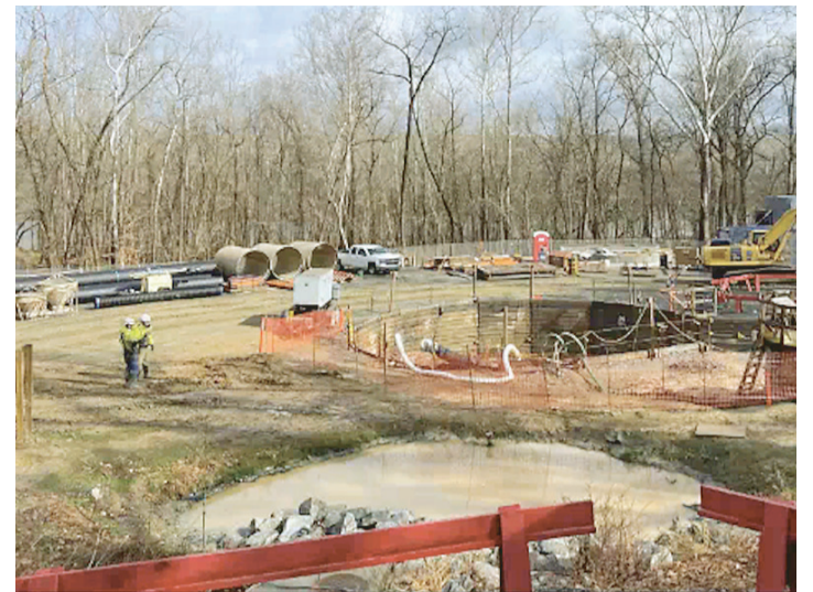
SCREENSHOT VIA LIVE FAIRFAX COUNTY VIDEO, DC WATER.COM Orange fencing encircles the initial affected area adjacent to Manhole # 31
