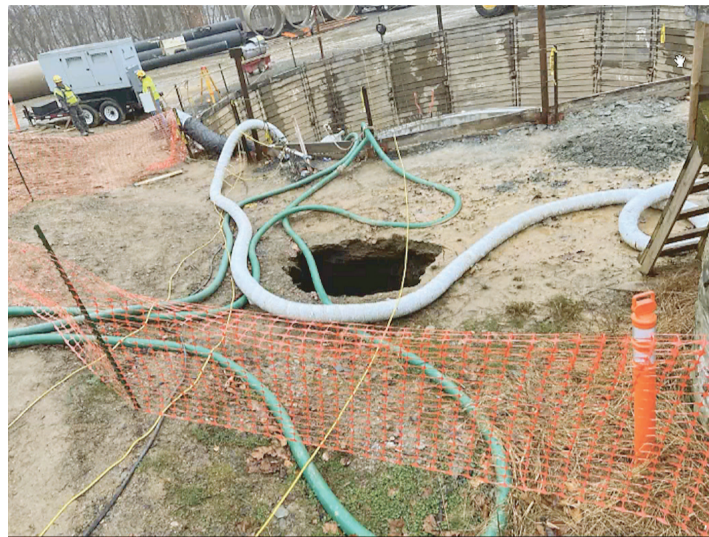
SCREENSHOT VIA LIVE FAIRFAX COUNTY VIDEO, DC WATER.COM Discovered Monday, February 12, the sinkhole at DC Water's Manhole #31 appeared small.
