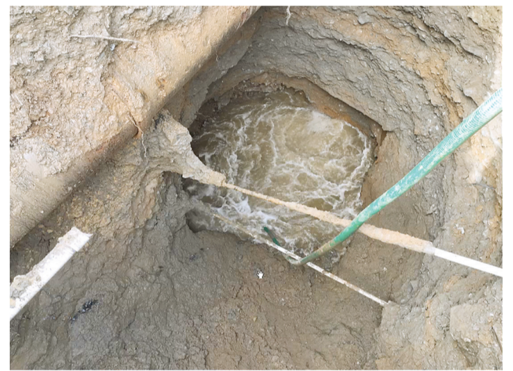
SCREENSHOT VIA LIVE FAIRFAX COUNTY VIDEO, DC WATER.COM A drone captures the image to identify the manhole collapse as sewage continues to flow through the breached pipe. At the time, DC Water reported no overflows.
