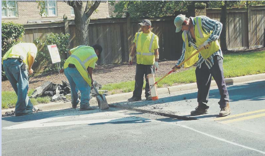
The county had the new speed humps in the Eldwick community repaired after finding they did not match design specifications.
