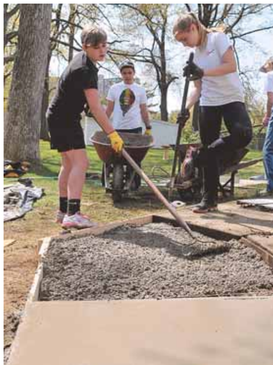
Volunteering with Fairlington United Methodist Church, Beck Moniz, Kate and Emma Sapp work on a filling a second slab of concrete for a homeowner in West Alexandria.
