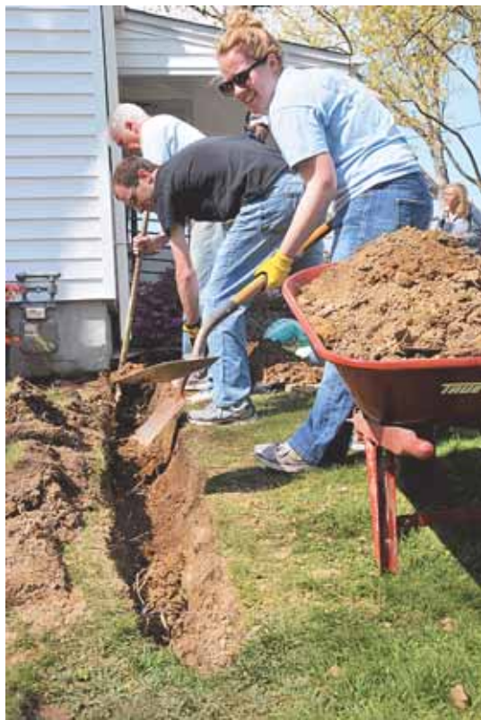
Allie and Dave Walker work to clear a gutter drainage ditch in a side yard.
