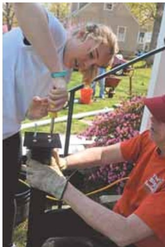
As Kent Smiley holds a handrail post, Jessica Killeen works screws into the support base for placement on the front porch.
