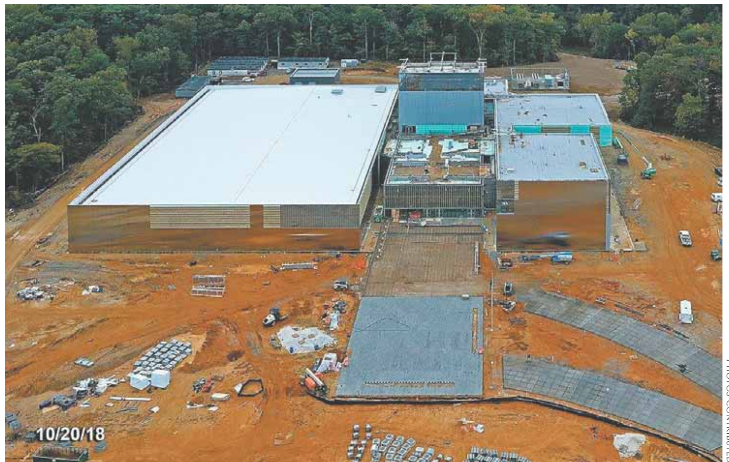
Construction crews have a majority of the outside completed, but there is much to do on the exhibits, artifacts and technology inside.
