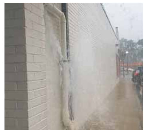
Waterworks, not fireworks. This drain pipe behind the Nail Salon and Chill Zone parking lot off Harrison was overwhelmed by the flow and sparked off a shower of water for more than an hour.
