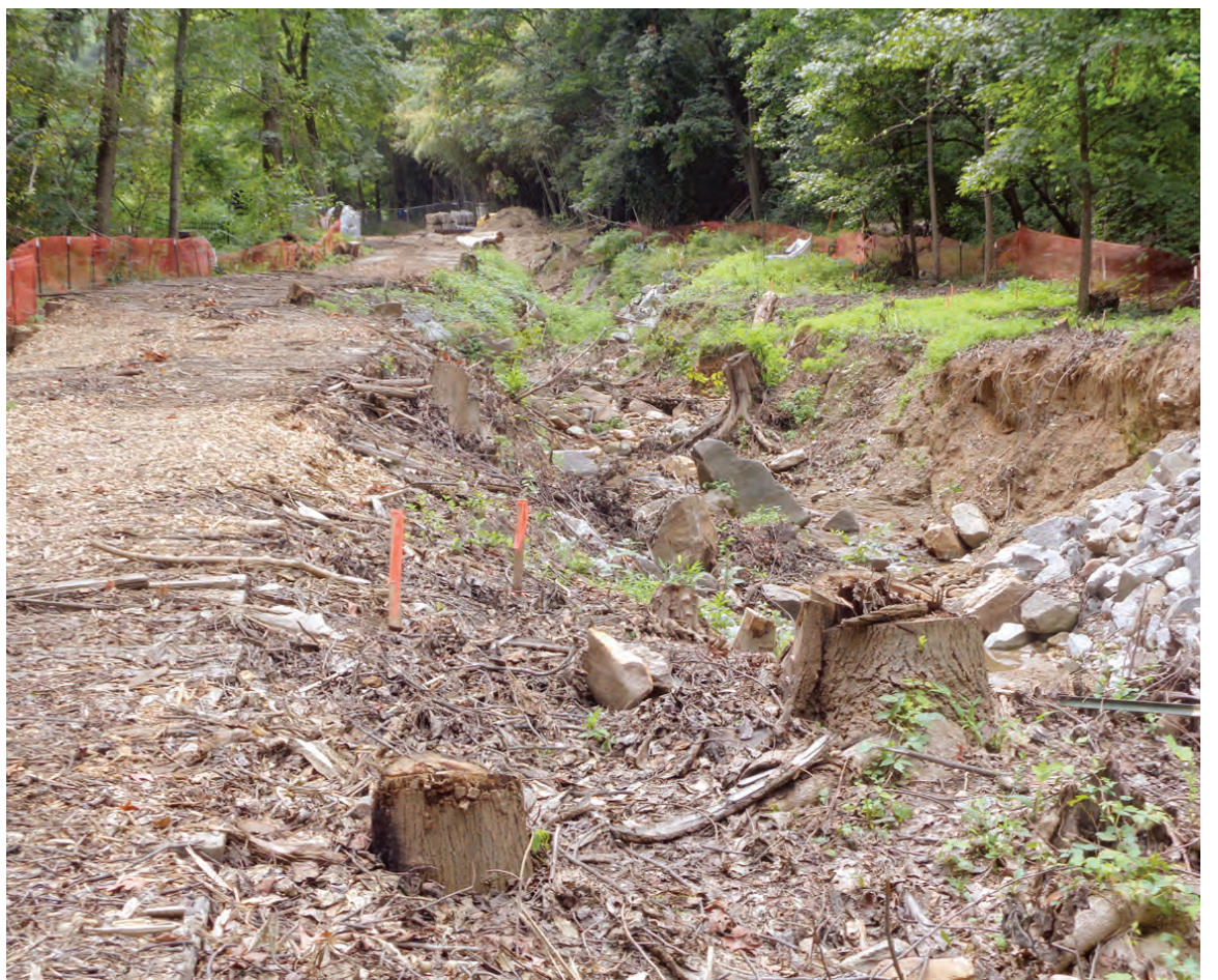
AFTER: Trib B of the Donaldson Run after the tree removal as the “restoration” process begins.
