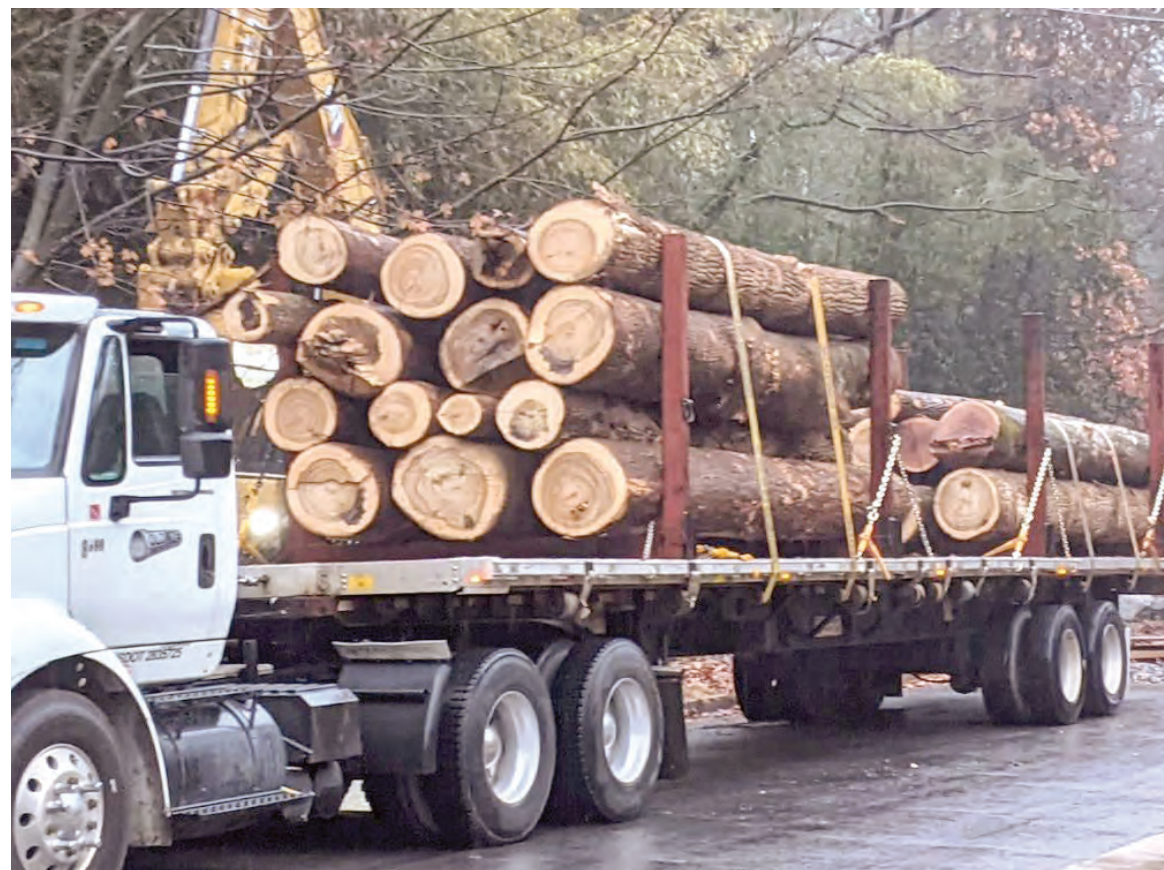
Some of the 86 mature canopy trees removed from the Donaldson Run Trib B stream being hauled away.
