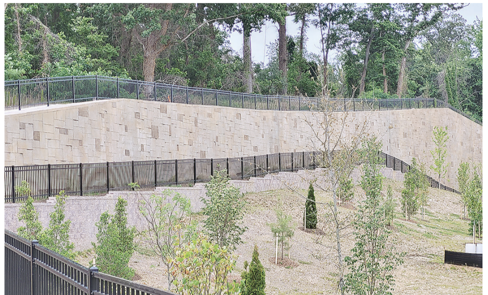
The wall to hold back the marine clay was a big part of the project.
