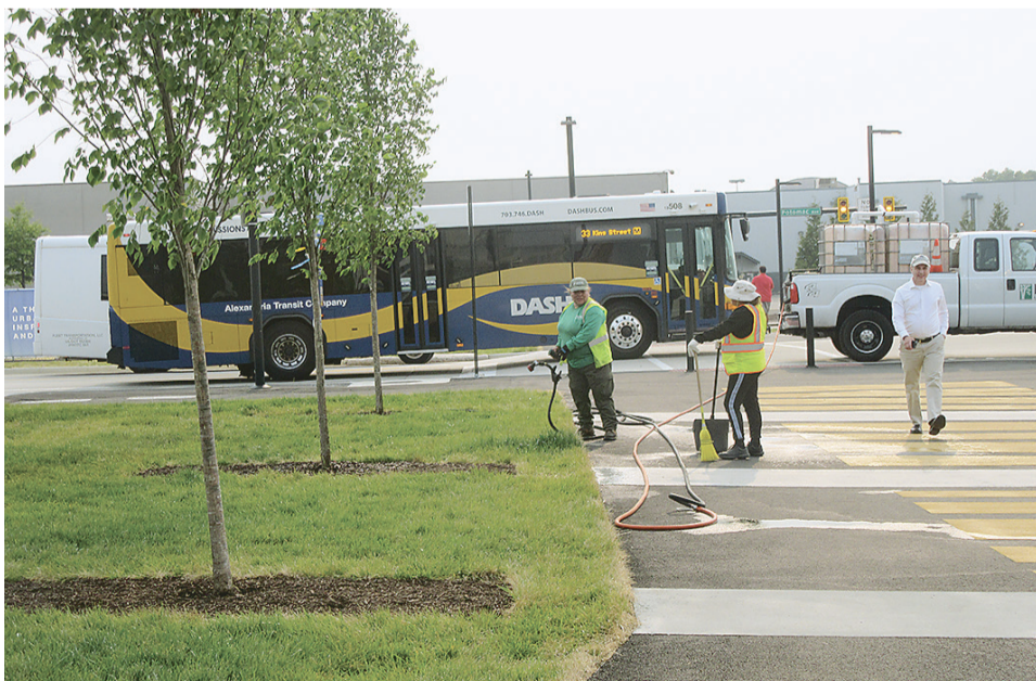
Workers are now putting in plants and trees. The DASH bus has a stop nearby.
