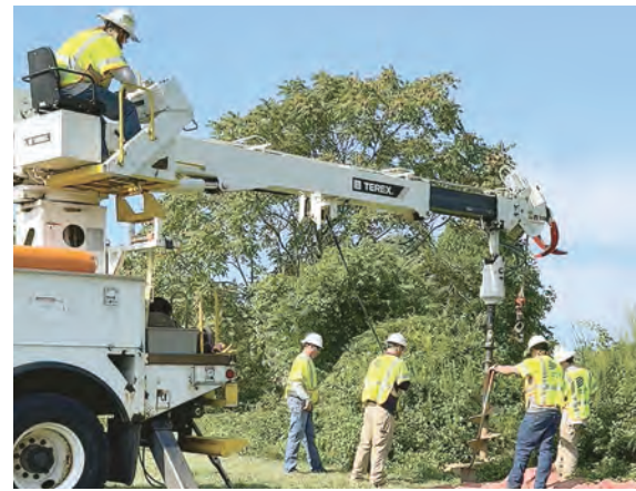
Ryce Zink operates auger to create deep hole to accommodate platform pole
