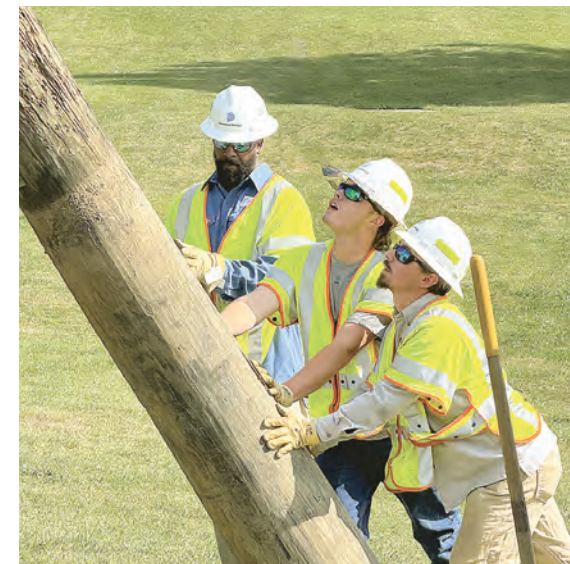
Ground crew members Andre Miller, Aiden Marshall and Bren Knight guide pole on winch to placement
