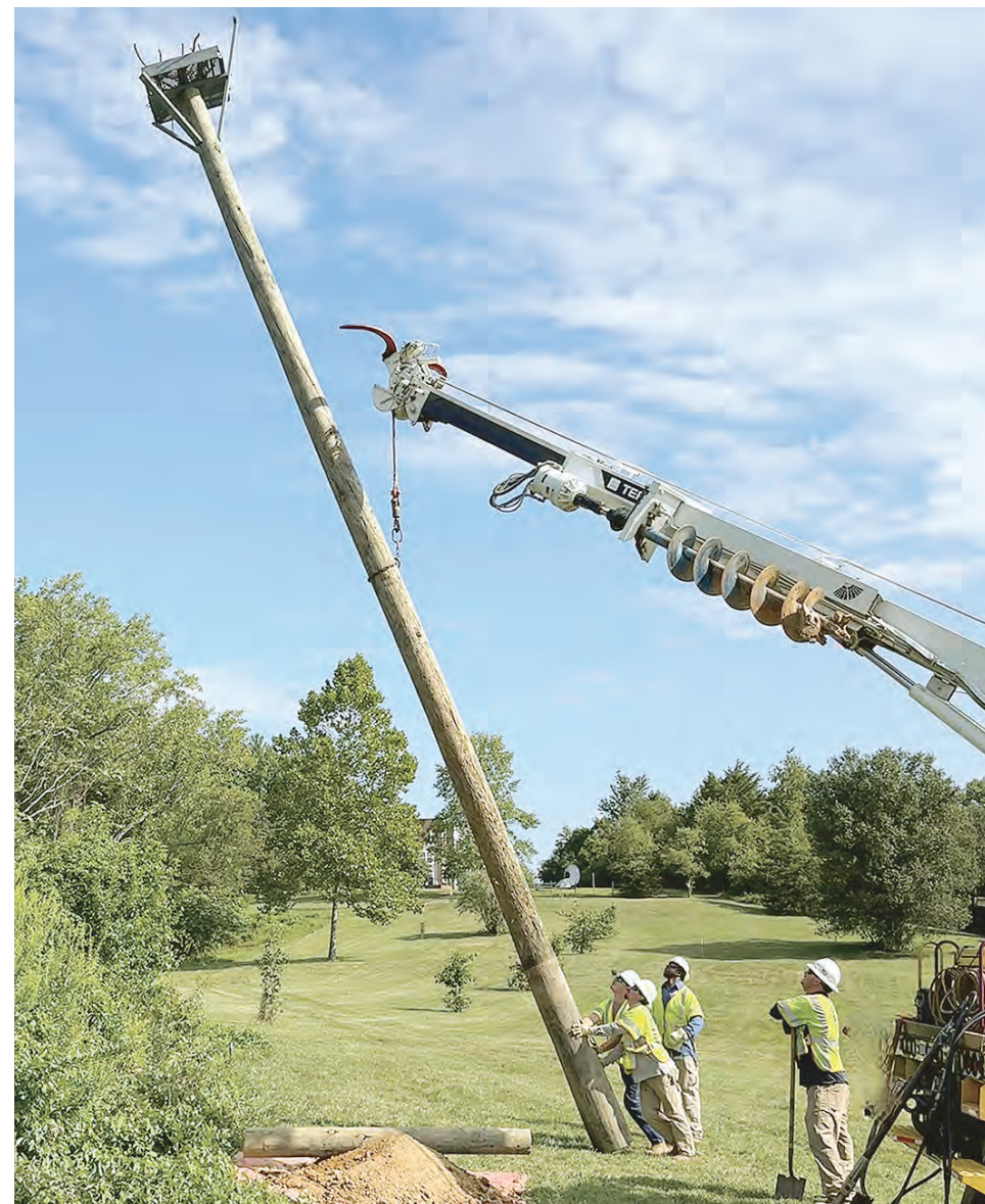
With auger retracted, the derrick with pole guides and winch maneuver the pole
