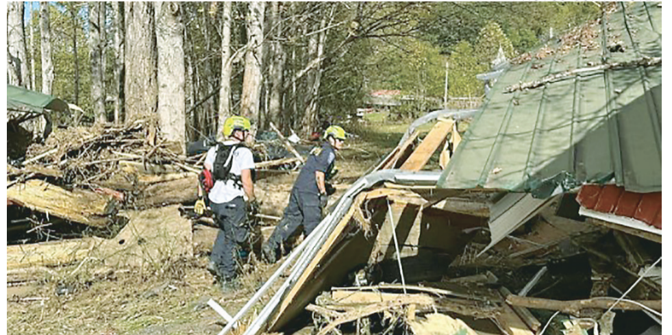
Flood waters caused this house to collapse.
